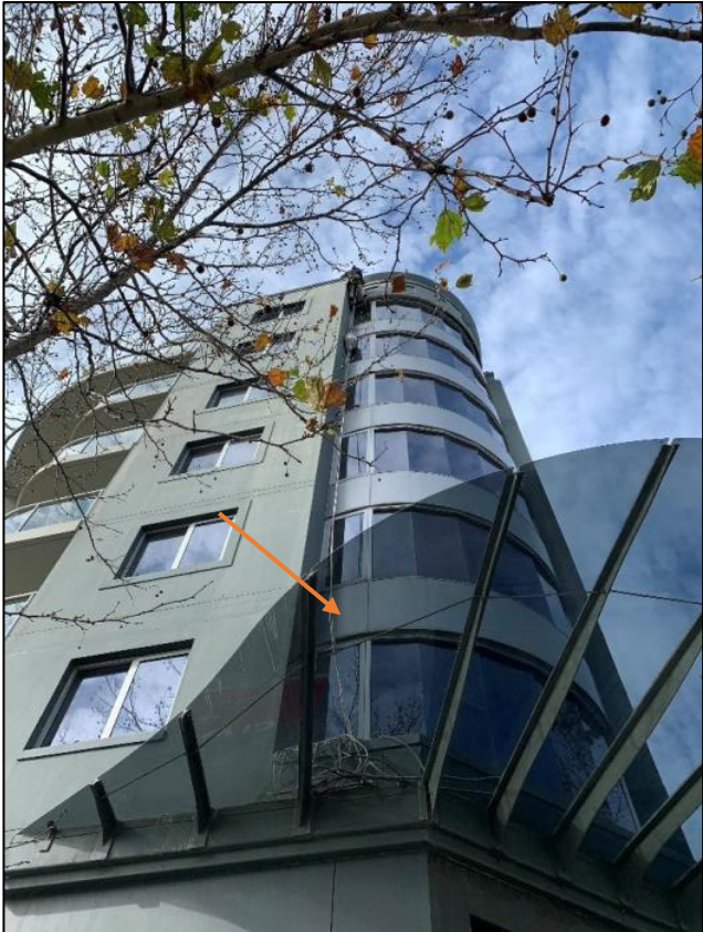
Photograph 3 – Location of sample (SW corner of the building) taken for laboratory testing
